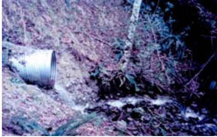
Outlet showing small undercut erosion site, side view, 04/06/99
