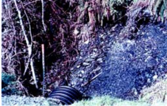
Typical 18" plastic ditch relief pipe also drains small springs from cutbank, 04/06/99
