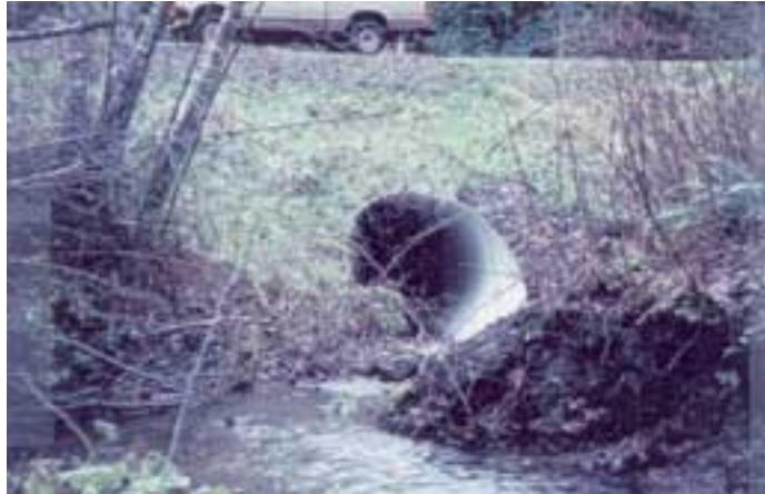
Inlet showing deposition at left after headcut migration, 01/10/01
