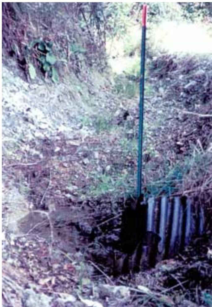
Inlet view, note ponding, 11/20/00
