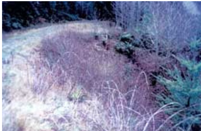
Outlet side view overgrown by vegetation, 01/10/01
