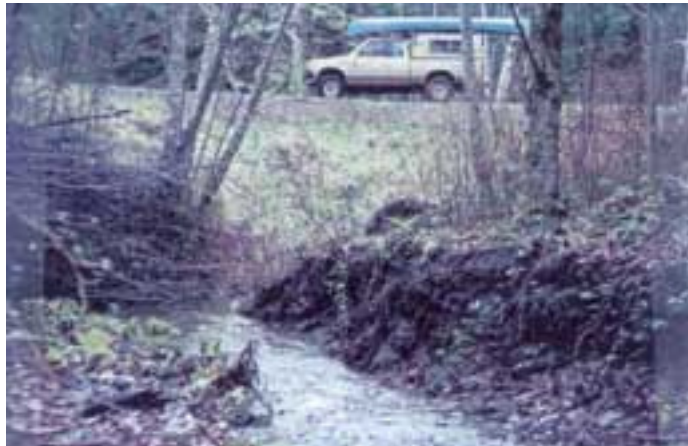
Inlet showing headcut, 01/10/01
