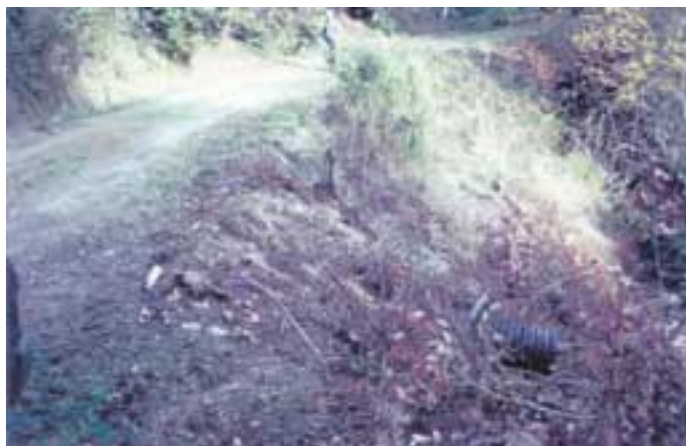
Outlet view, note cracking along edge of fill, 11/20/00
